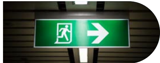
EMERGENCY AND SAFETY SYSTEMS
